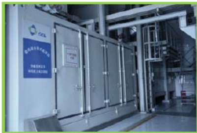
ZK1200 Gas Turbine Set
