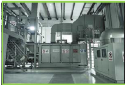
ZK1200 Gas Turbine Set
