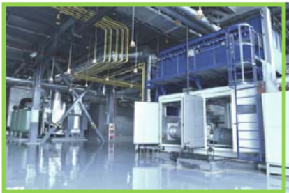
ZK1200 Gas Turbine Set
